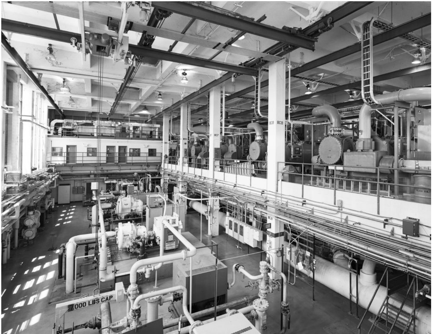
Kansas City Plant power house, 2013 (Historic American Engineering Record, U.S. Department of the Interior/Richard Welnowski)
