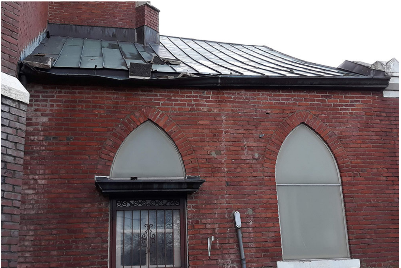
Sacristy roof damage at Assumption Church in Nashville, caused by the March 3 tornado (Mark Cassman)
