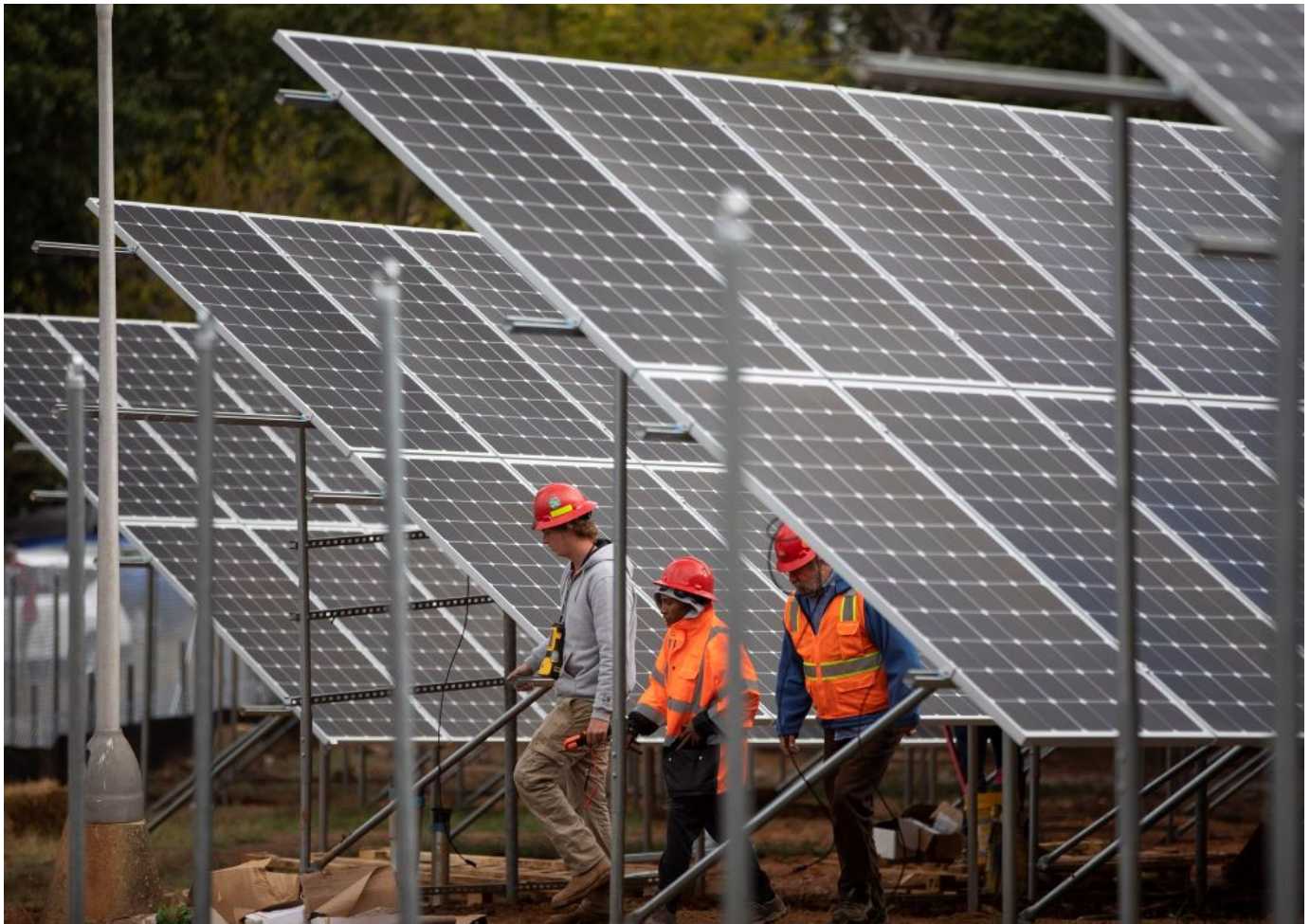
Workers in Washington are seen near solar panels Oct. 17, 2019, on the property of Catholic Charities of the Archdiocese of Washington. (CNS/Catholic Standard/Andrew
