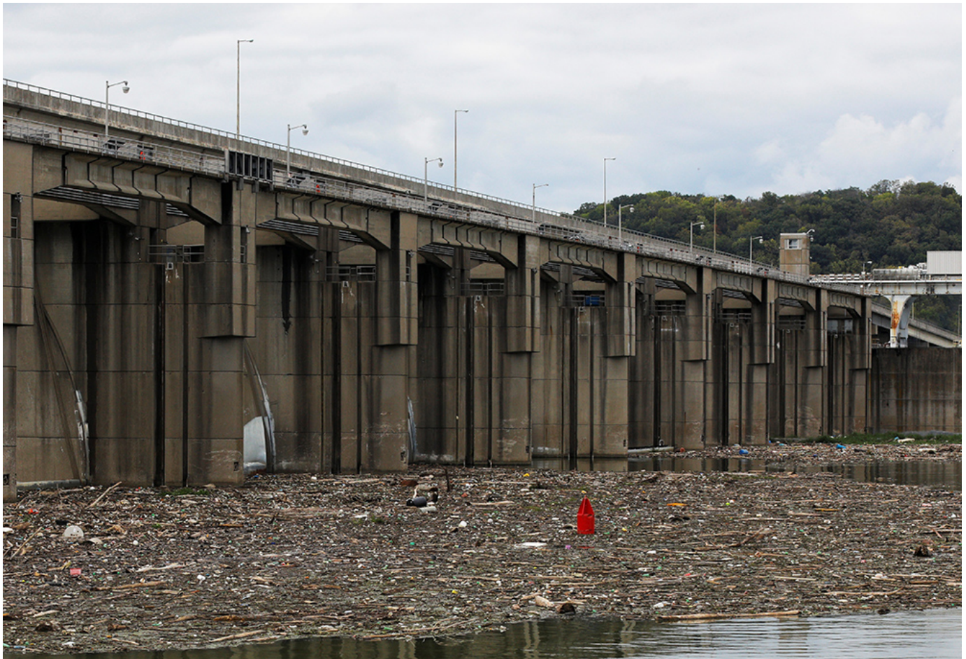
Garbage and debris pile up behind the Markland Locks and Dam on the Ohio River Sept. 14, 2017, in Florence, Indiana. (CNS/Reuters/Brian Snyder)
