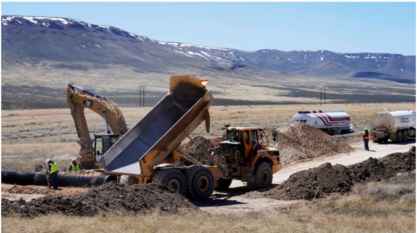
Construction continues at the Lithium Nevada Corp. mine site Thacker Pass project on April 24, 2023, near Orovada, Nev. (AP/Rick Bowmer)
