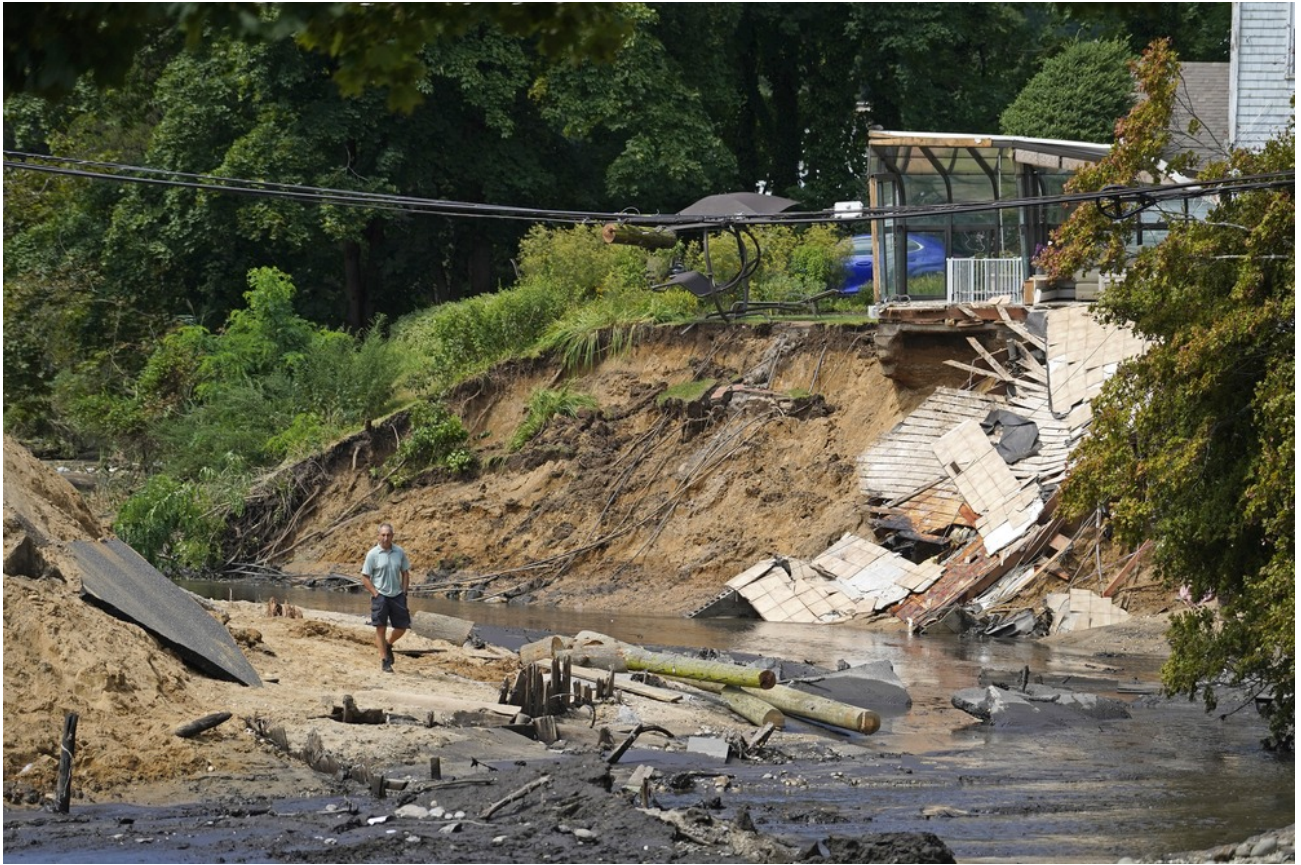
A man walks on the dirt and sand foundation of Harbor Road in Stony Brook, N.Y., Aug. 19, 2024, after it collapsed earlier in the day when torrential rain caused a dam beneath the road to burst. The storm unleashed flash floods in parts of Long Island, N.Y., and southwestern Connecticut, where two women were found dead after they were swept away from their vehicles. (OSV News/Gregory A. Shemitz)
